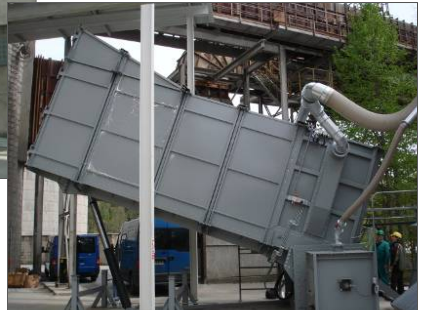
Container placed within fully enclosed vented enclosure
